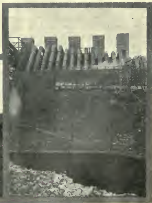
LOWER END OF COOLING PIPES.
